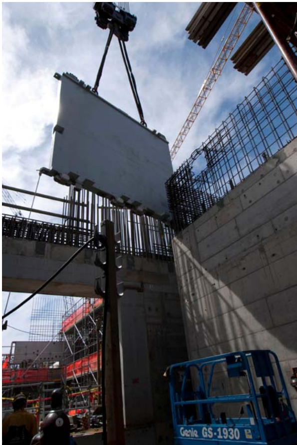
A 50-ton shield door requires precision installation at the High-Level Waste Vitrification Facility at the Hanford Waste Treatment Plant.
