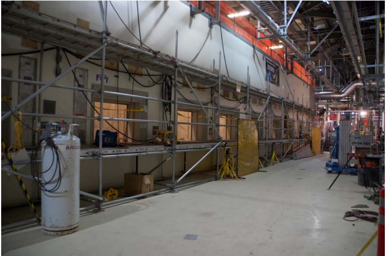
An integral component of WTP's Analytical Laboratory (Lab), the waste transfer system is being installed at the far end of the Lab hot cell area.
