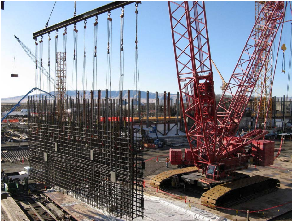
The more than 36-ton rebar curtain was installed on the fourth elevation of the Pretreatment Facility. The fourth elevation brings the facility's height to 77 feet.
