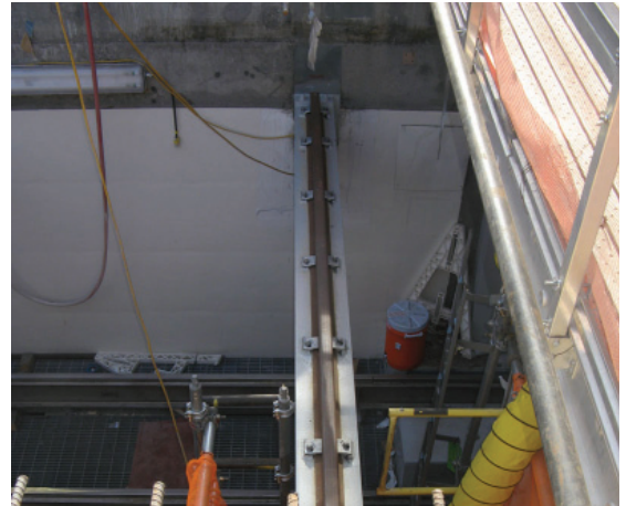
The crane rails will transfer large carts used to transport full waste canisters.
