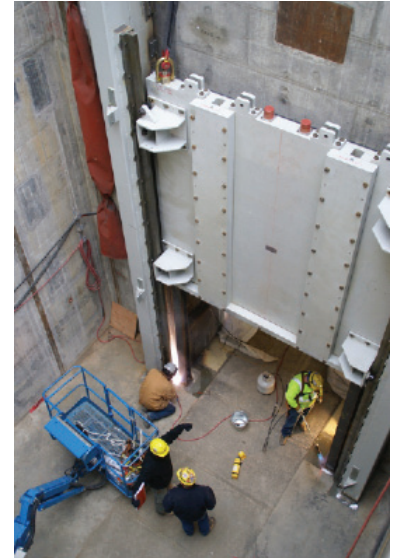
The cask lidding door, like the drum lidding room door, is 10 feet high, 22 feet wide and approximately eight inches thick. These doors will provide radiological shielding protection to workers when the vit plant is operational.
