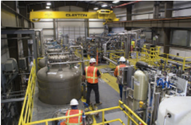
The Pretreatment Engineering Platform is a quarter-scale demonstration facility that is confirming the efficiency and throughput of select pretreatment processes.
