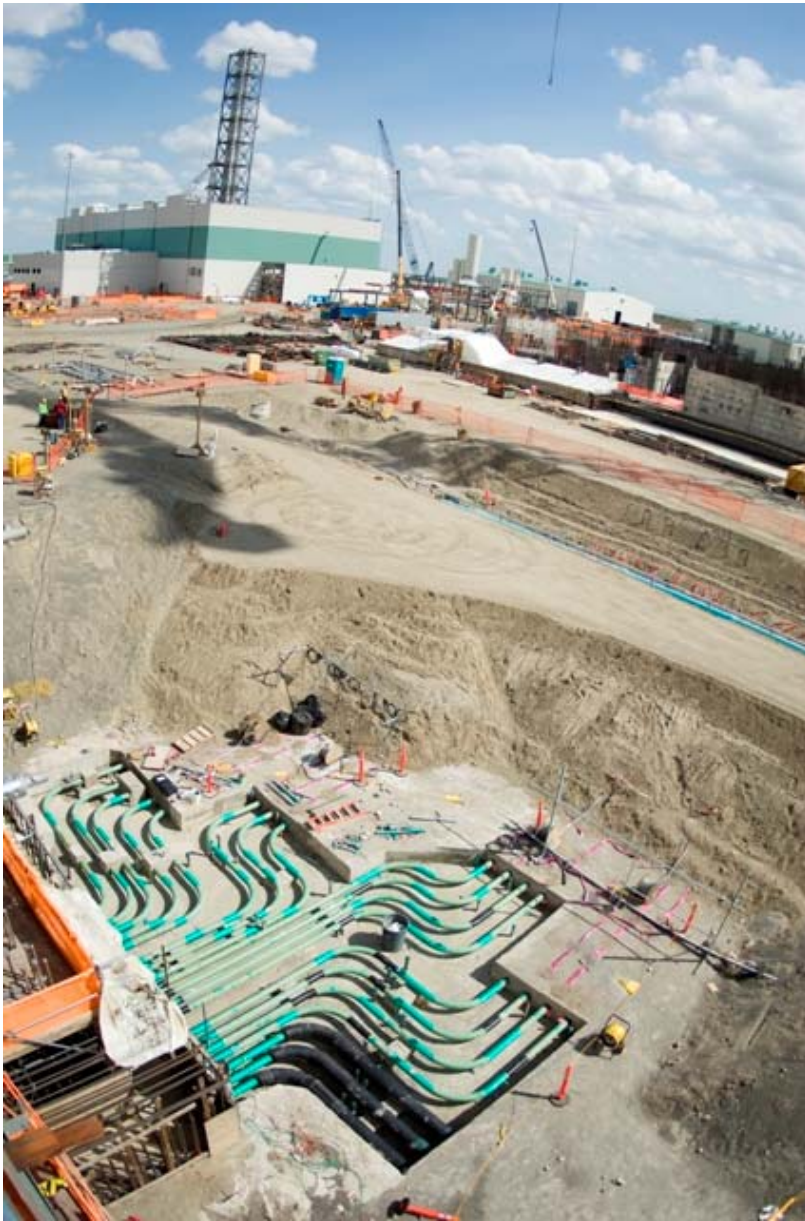
Photo caption: A view of the cathodic protection system, last April, before it was backfilled.
