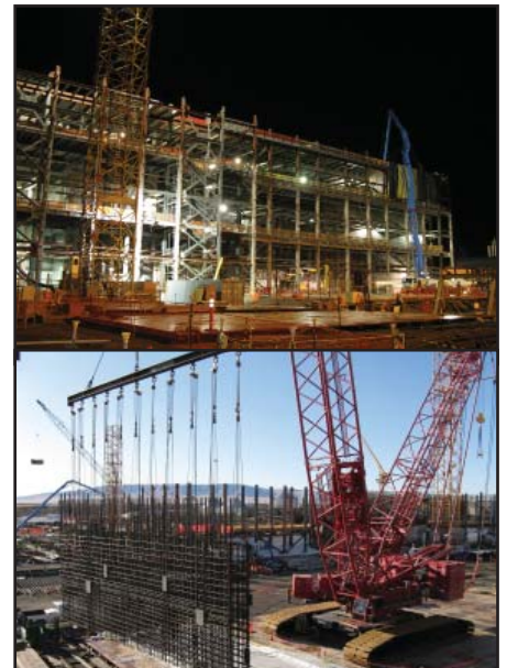
Top: A concrete pump truck (far right) is used to place the 77-foot elevation concrete. Bottom: The 36-ton rebar curtain is lifted by the Demag crane.
