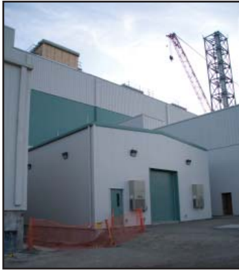
The switchgear building equipment will serve as the facility's primary power source.
