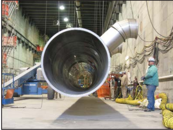
The HVAC duct is five feet in diameter and, when completely installed, will span the length of the 400-foot hot cell.
