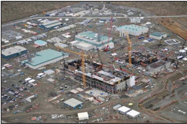
The WTP Project finished 2009 at 52 percent complete and with the best safety record since the project's inception in 2001.
